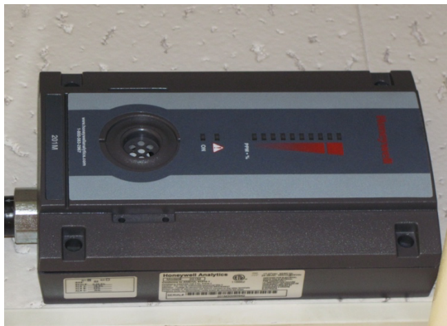
Figure 4 – Example of an oxygen sensor located (room EB-44).
